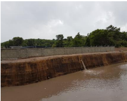
TenCate Polyfelt® Envirofelt CF350 covered reinforced soil slope surface to enhance vegetation growth
