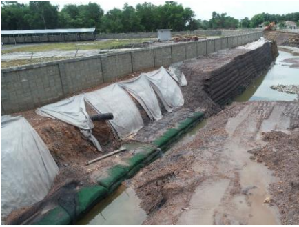
TenCate Geotube® geobag placed at the bottom of reinforced soil slope with TenCate Miragrid® geogrid
