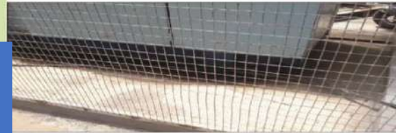
Genset within concrete bund at plot 37
