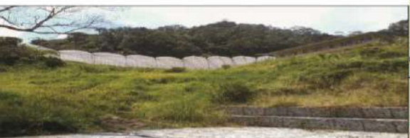
Slope at RP4 is hydroseeded and stabilised with gabions encased in wire mesh
